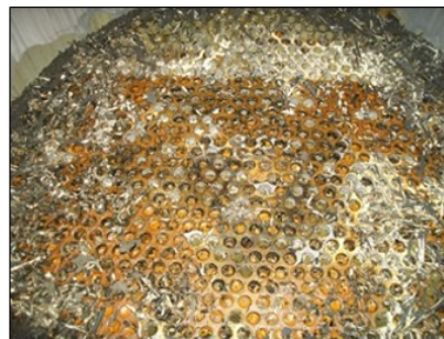
Evaporator Prior to Treatment
