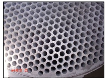
Evaporator After Treatment With Solenis Program
