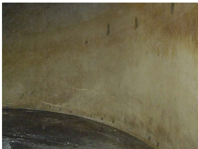
With the Biobond Program: whitewater chest walls clean, no deposition
