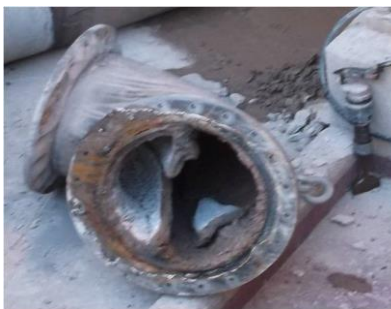
Treated tank/feed pipe – easy to break apart scale, less total deposit, 5% obstruction of flow after 6 weeks
