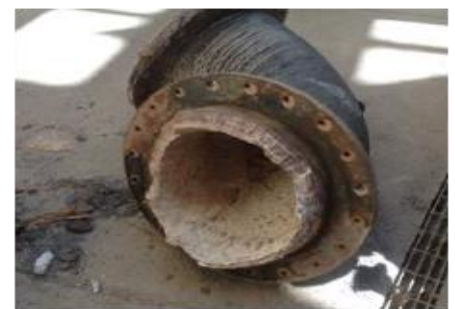
Untreated tank/feed pipe – hard to break apart scale, more total deposit, 40% obstruction of flow after 6 weeks
